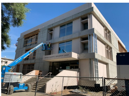
Renovations under way for the Center for Quantum Mathematics and Physics in the former Physical Sciences and Engineering Library.
